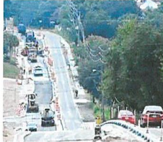
PAUL CRATE | LEDGER MEDIA GROUP Paving has begun just north of State Road 544 in the northbound lane of the State Road 17 road improvement project that runs from SR 544 to Hinson Avenue in Haines City. The project is expected to be completed in the summer of 2015.
